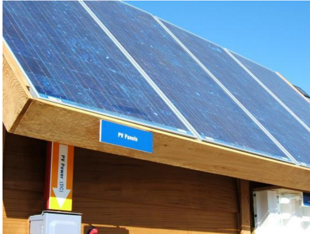
Photovoltaic array. 2007 Solar Decathlon, Washington, DC. Photo by author.
