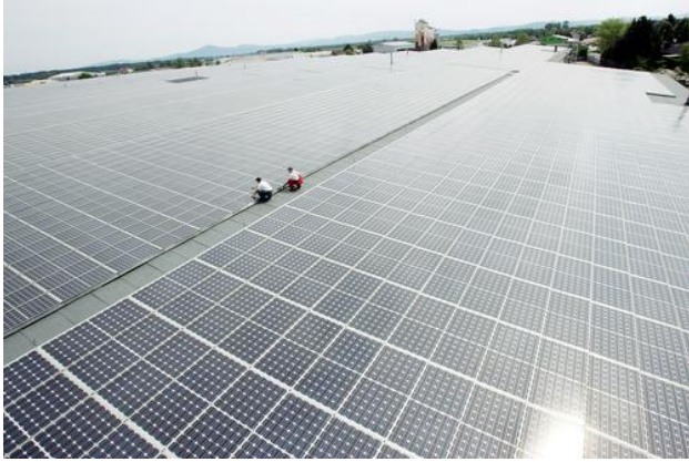
Buerstadt, Germany: The roof of a warehouse, equipped with solar panels, May 13, 2005. The 50,000 square meter system with a capacity of 4.5 megawatts per year represents the largest roof based solar system worldwide. Photo by Ralph Orlowski/2005 Getty Images, Inc.
